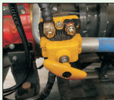
Battery Cut-Off Switch
